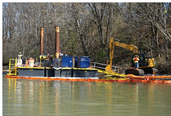
Figure 3.52. Workers excavate soil from the EU-19 mudflat to load on the floating platform
