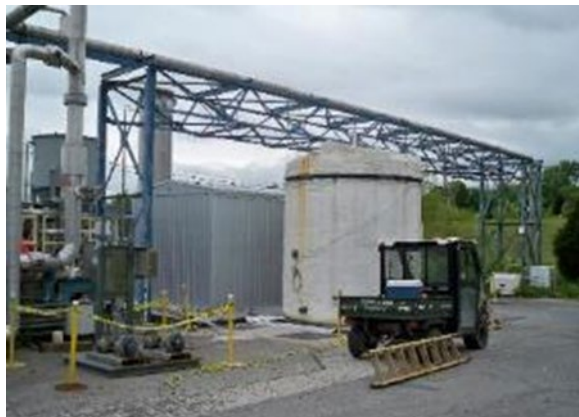
Figure 3.16. The Chromium Water Treatment System
